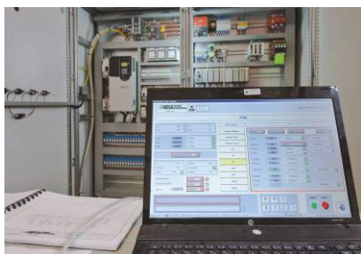
The electrical panel with a view on the PLC control system software.
