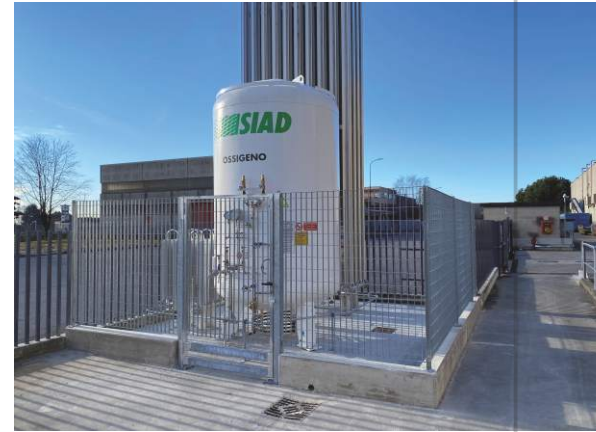
Oxygen tank with evaporator
